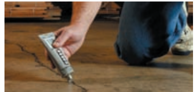
Seal cracks in cement floors.
